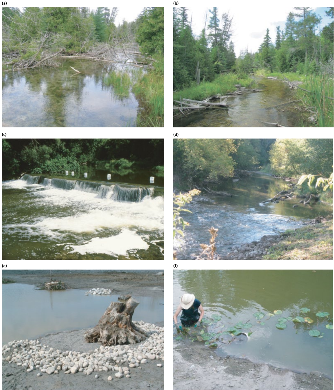
Figure 6.3.4 Various restoration strategies including (a) before and (b) after debris removal and structure placement in a stream, (c) before and (d) after dam removal on a stream and (e) construction of habitat structures in a dewatered embayment of a lake and (f) the subsequent planting of endemic vegetation in littoral habitats of a newly created embayment.
